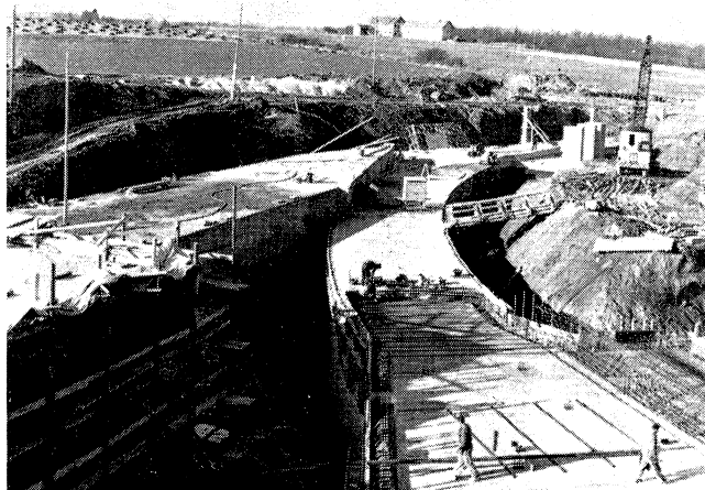
Above is a view taken during the construction of the PS, showing the ring tunnel and the linear accelerator wing (left) before the concrete structure was covered with earthfill. The photo on the right shows the 50 MeV linear accelerator tanks (30 m long) being aligned. The output end is in the foreground.
