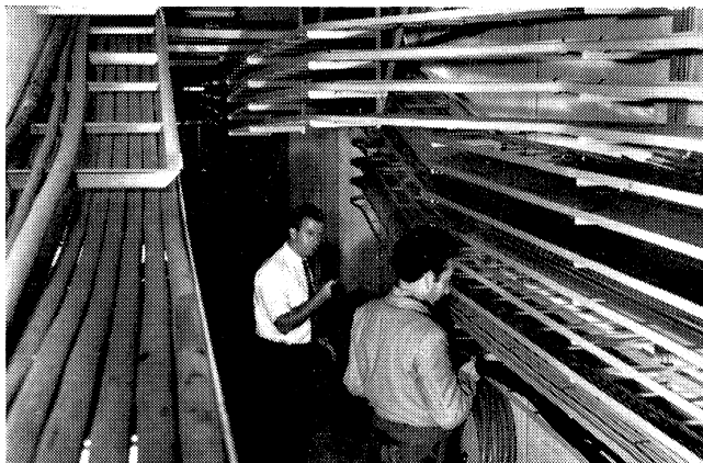
The PS magnet blocks (right) were stored in the South Experimental Hall prior to their assembling in 10-block units. Below is a view of the intricate cabling system running underground. In the PS, cable length amounts to some 3 600 km.
